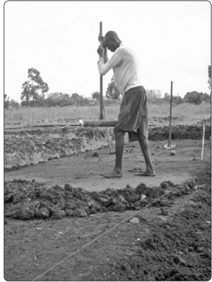
Figure 2.2-6. Dyke construction is done in layers about 20 cm thick. Each layer is well compacted before the next layer is added.
