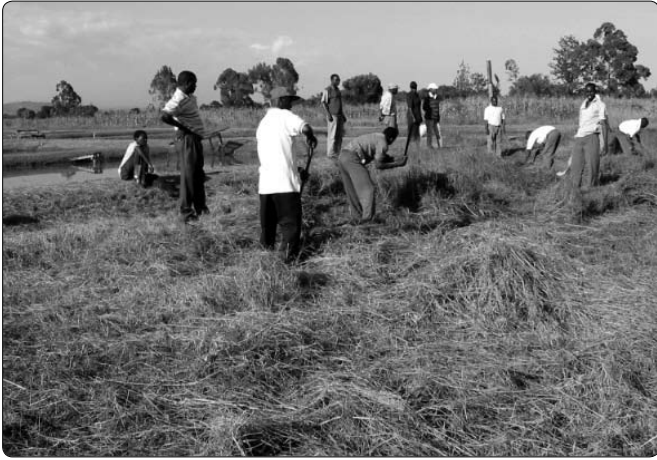
Figure 2.2-1. Vegetation and topsoil should be removed from the area before beginning to build a pond.
