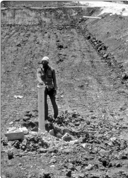
Figure 2.2-7. A PVC standpipe being installed in a new pond. With the standpipe in the vertical position the full pond will have a water depth of approximately 1 m.
