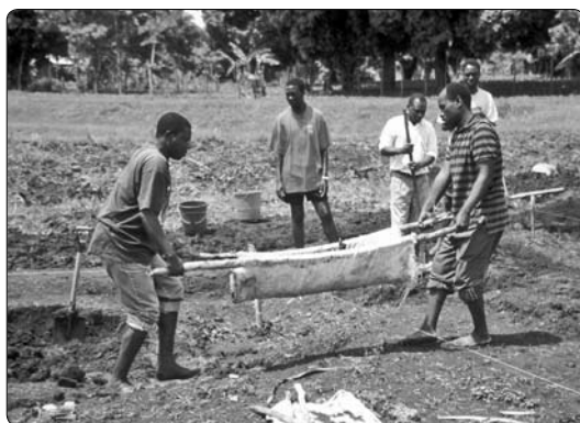
Figure 2.2-5. A two-person stretcher works very well for moving soil from the excavated area to the embankment area, especially in heavy clay soils.
